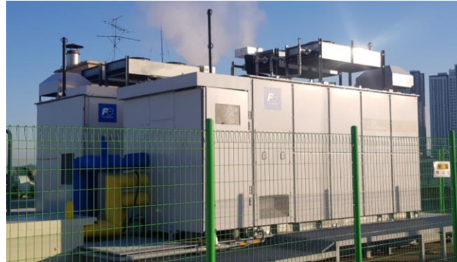
Leisure Town. power plant, 100kW
