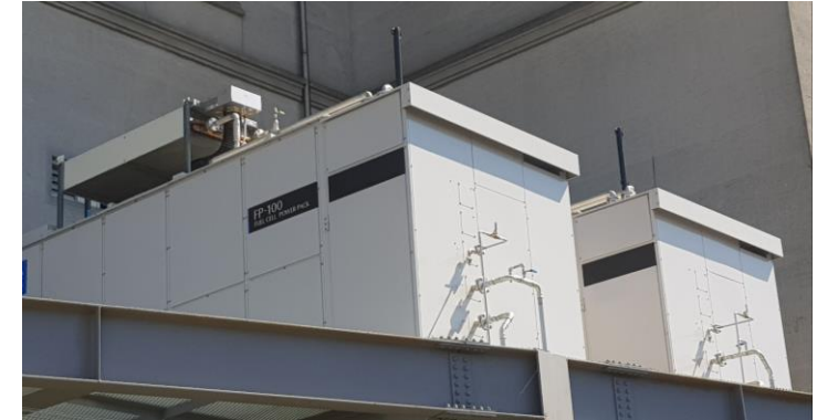
Hospital. Power plant, 200kW
